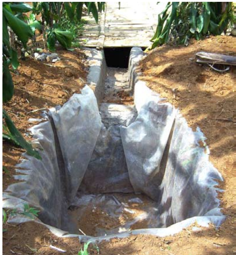
Quality well The quality of these wells is excellent. The farmers are careful to seek out and use only the best materials, including gravel, natural fibers, and plastic.
