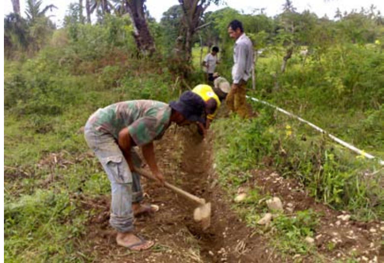
Pipe is on A strong camaraderie in Keutapang leads to a new water facility for the entire village
